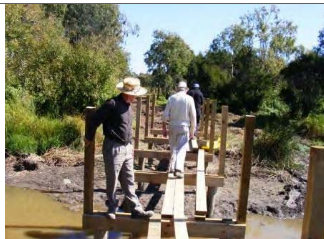
Walking the plank on next section of board walk under construction (piles & cross heads now complete on all four sections) following inspection John presented a $30,000 cheque to the Club the 1 st drawdown on his $100,000 contribution
