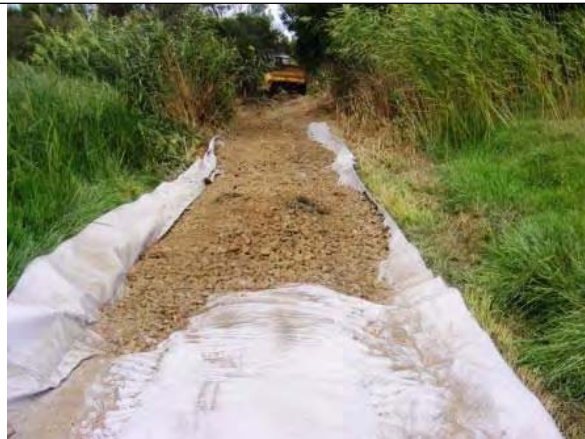
The same section two hours later with geofabric laid and 30mm crusher run spread
